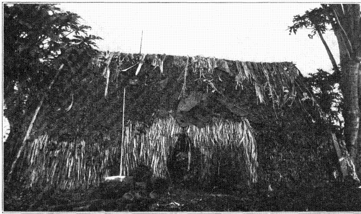
FIG. 83. HOUSE NEAR HILO NEEDING A NEW ROOF.
