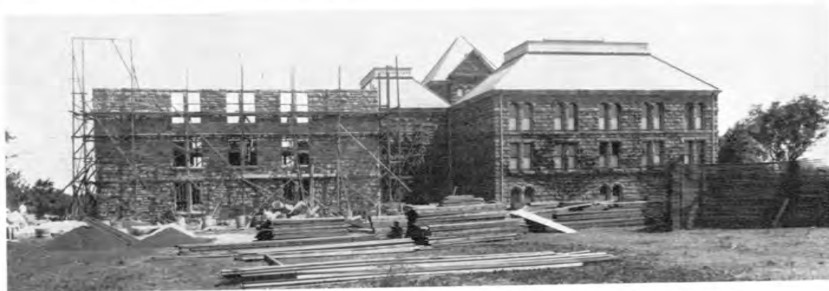
Rear view of Museum showing Hawaiian Hall under construction, 1899, opposite Polynesian Hall (right). Designed by Ripley and Dickey, the building was erected by Arthur Harrison for approximately $62,000 and paid for by Mr. Bishop. The frame house originally built for Principal Oleson in 1886 had to be moved 100 feet to the left to accommodate the new annex. Photo attributed to W. T. Brigham.
